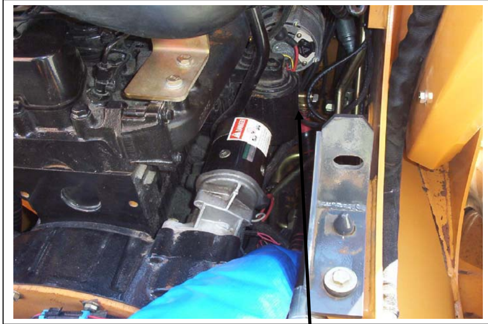
Water lines looping down under the engine and connected to heater tap.
